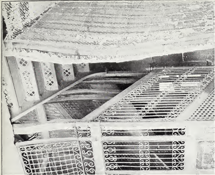
B. WARPING OF PLASTERED METAL-LATH COVERING BY FIRE, MURPHY BUILDING, SAN FRANCISCO. Photograph by Richard L. Humphrey.
